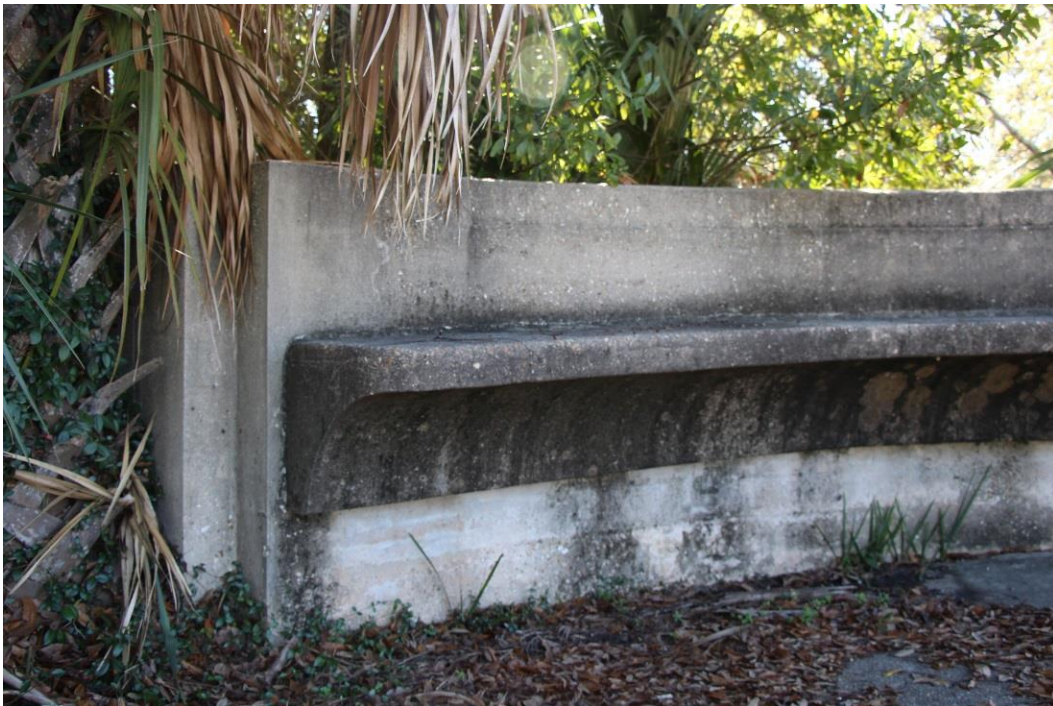
Condition Photo 1: Debris, vegetation, and mold/mildew on underside of integrated bench (northeast corner of Recall No.102235 shown).
