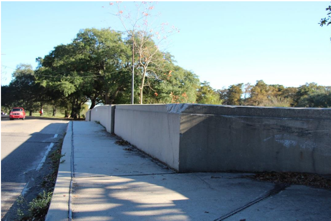
Condition Photo 9: Vehicle impact damage to concrete parapet/railing on integrated wingwall in southwest corner of Recall No. 102115.
