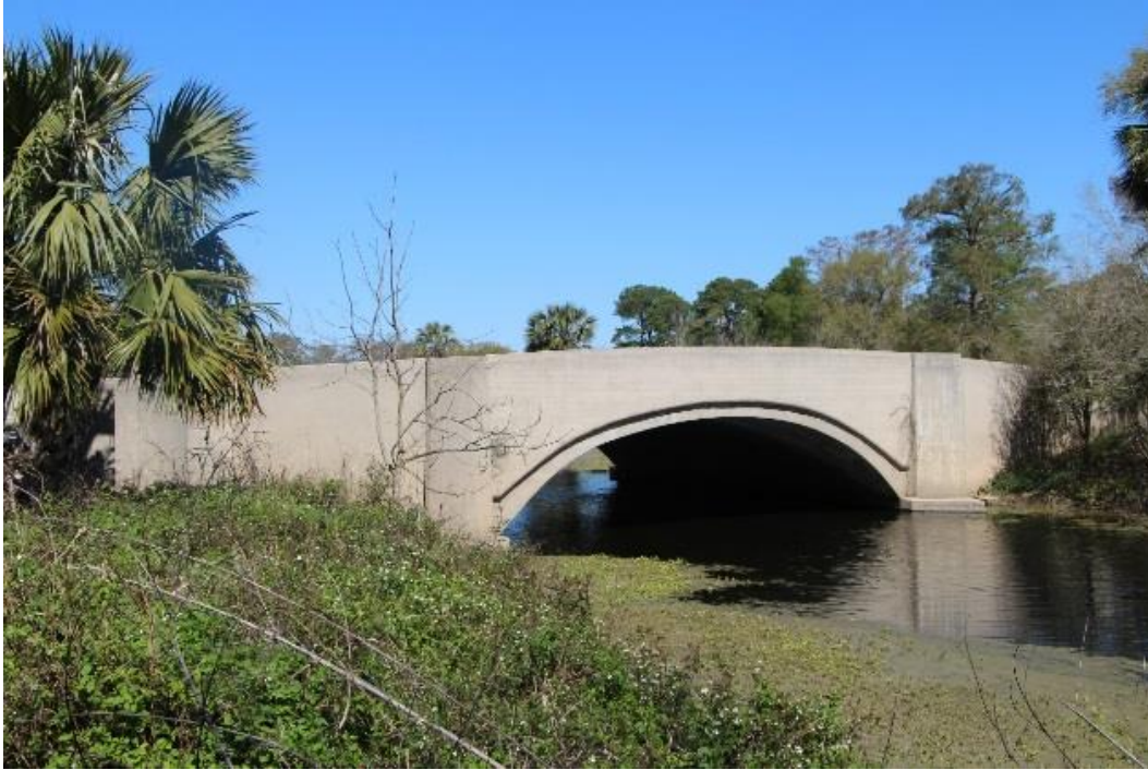
Character-defining Feature Photo 1: Design and construction of a closed-spandrel, reinforced-concrete arch with integrated curved wing walls and recessed arch ring (Recall No. 102237 shown).
