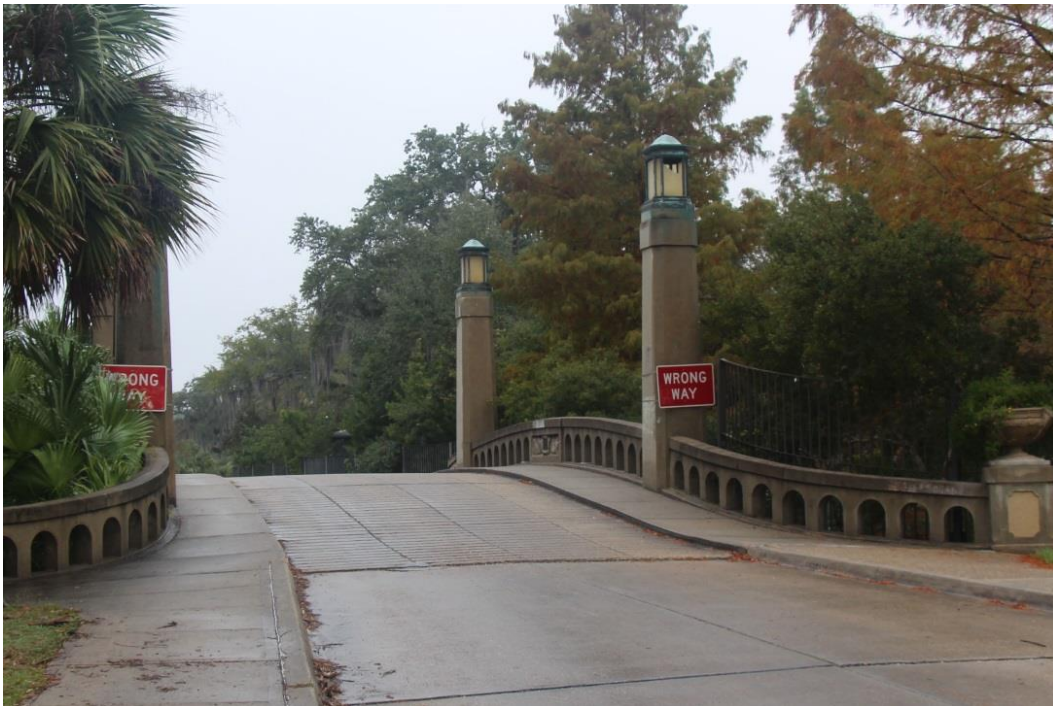
Condition Photo 11: Broken glass in northwest lamp post lantern on Recall No. 102227; condition of lights in four corners of the bridge is unknown.
