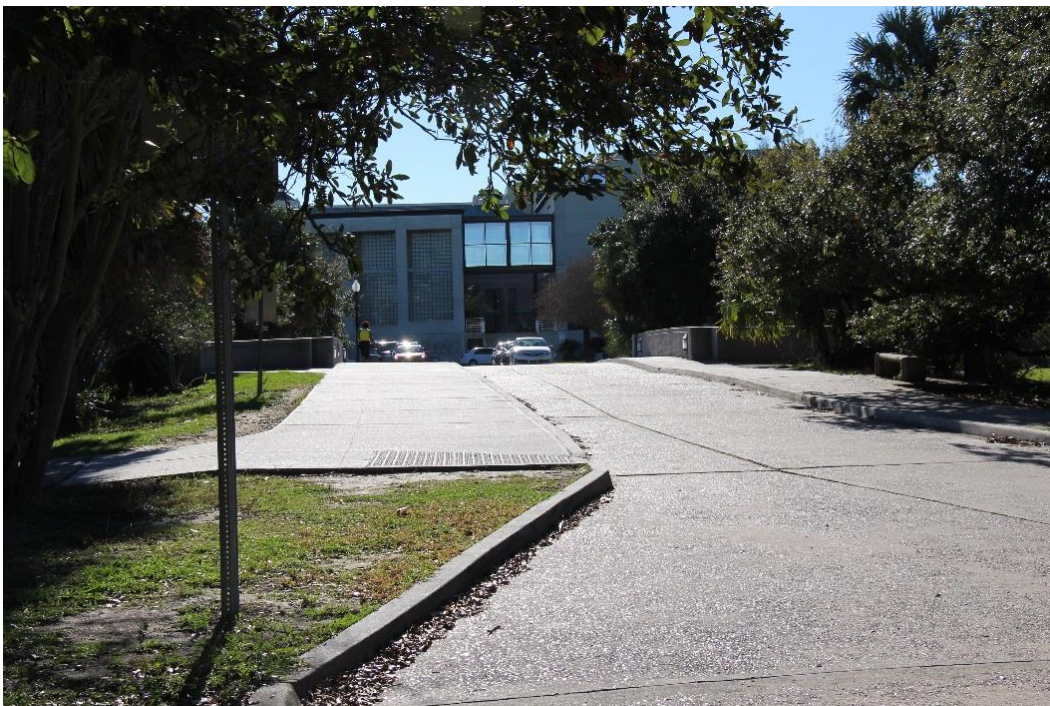
Condition Photo 15: North approach roadway of Recall No. 102233 with unsealed jointed pavement.
