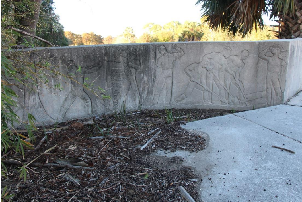
Condition Photo 2: Debris and vegetation accumulation and mold/mildew on concrete surface of bas-relief sculpture (southwest corner of Recall No. 102237 shown).
