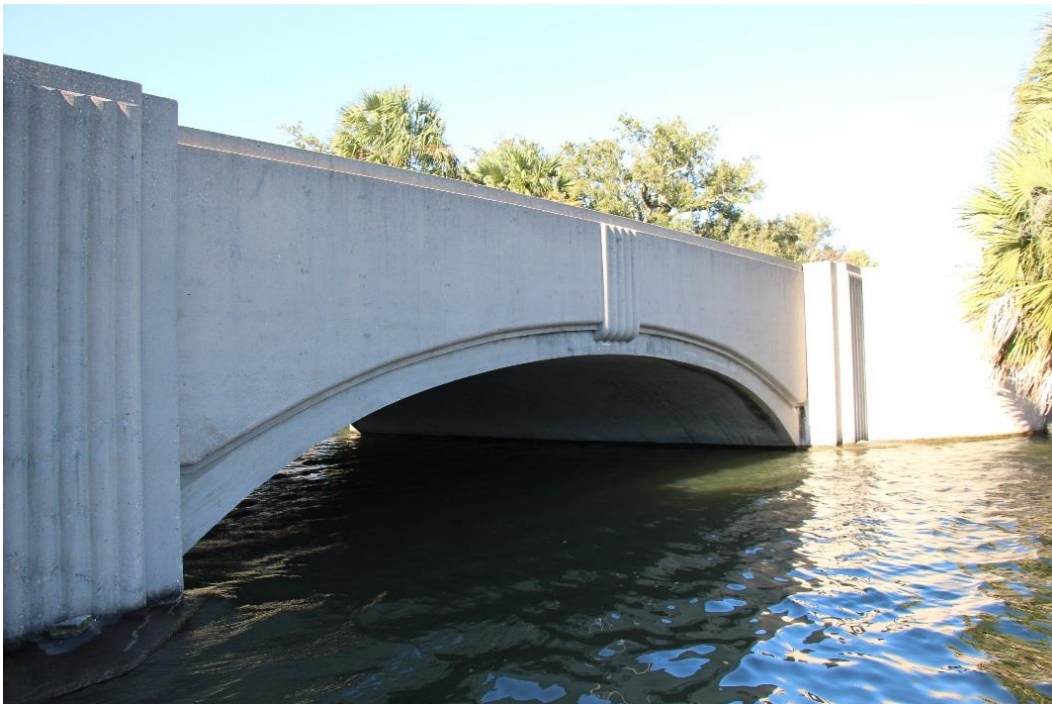
Condition Photo 13: Spalled and delaminated concrete on underside of arch of Recall No. 102233.
