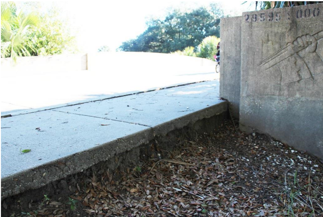
Condition Photo 21: Erosion in southwest corner of Recall No. 102236 at sidewalk, typical on all four corners of bridge.
