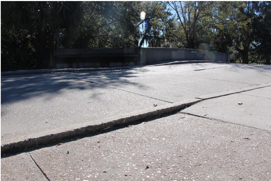
Condition Photo 19: Unsealed joints and settlement of roadway slabs at ends of Recall No. 102235, typical each end.
