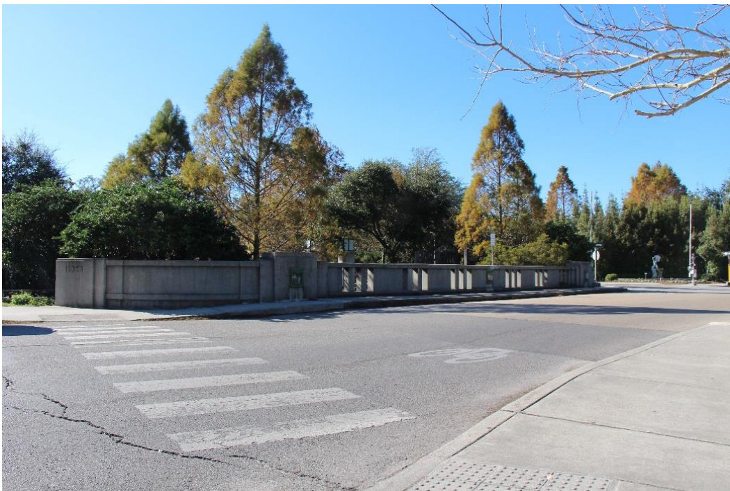
Condition Photo 17: Crack in west asphalt approach roadway to Recall No. 102234.
