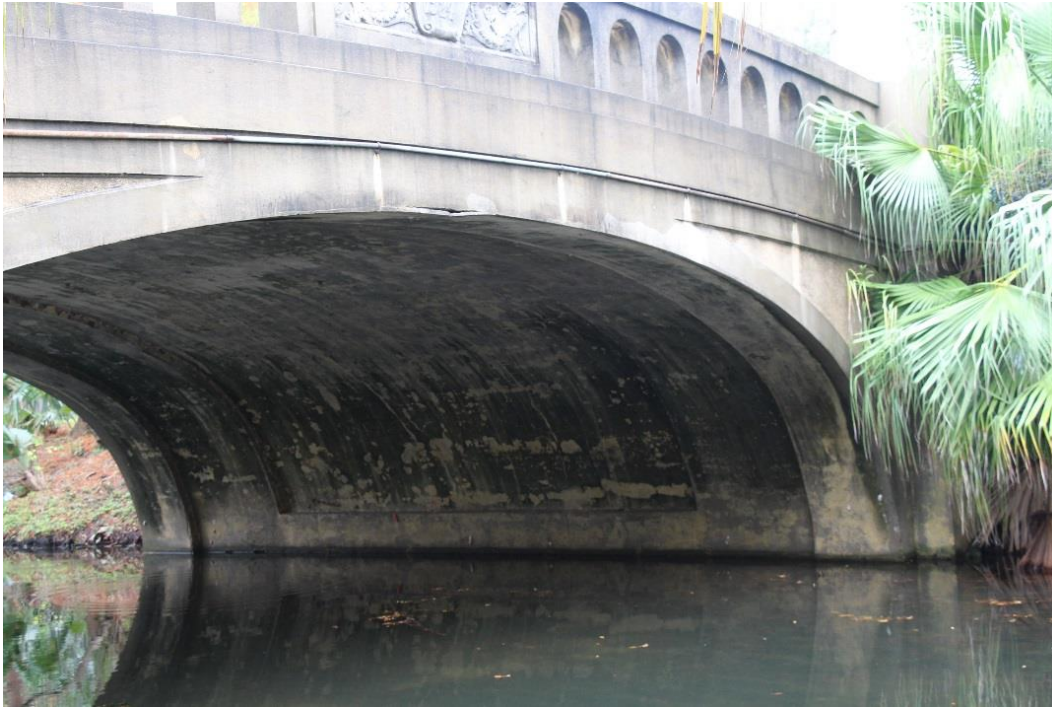
Condition Photo 12: Spalled and delaminated concrete on underside of arch of Recall No. 102227.
