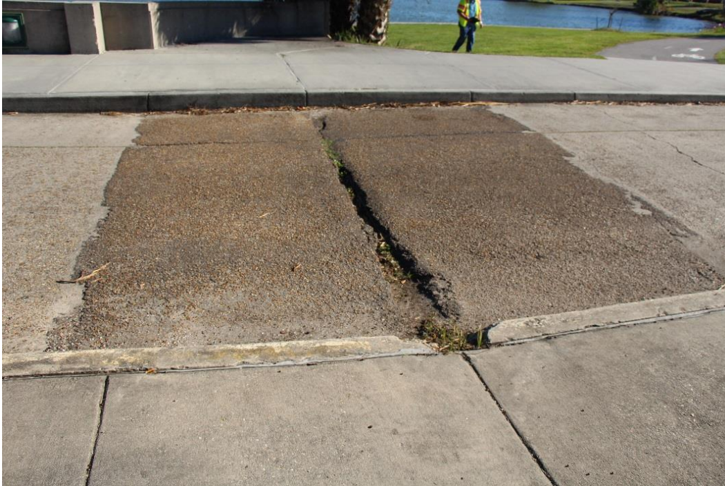
Condition Photo 14: Deteriorated and failed roadway pavement at south approach to Recall No. 102233.
